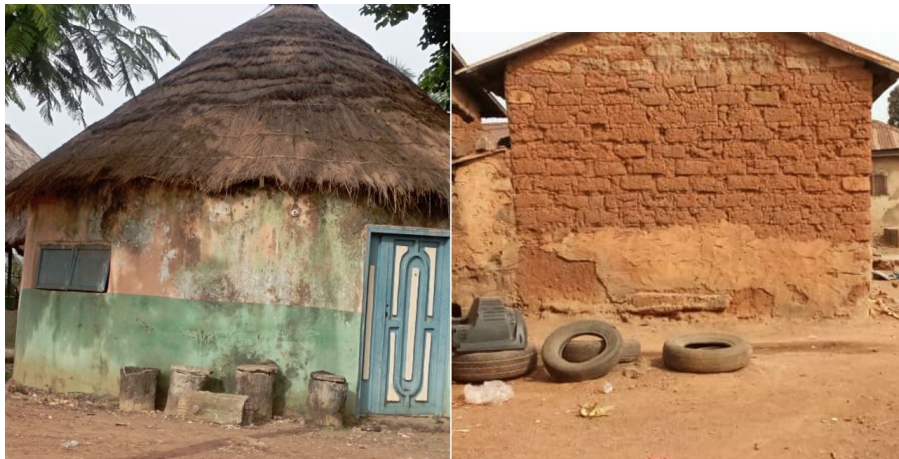
Figure 1. A typical example of mud buildings in Tammah and Gunki, Nasarawa, Nigeria.
